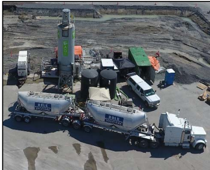
CDSM Batch Plant
